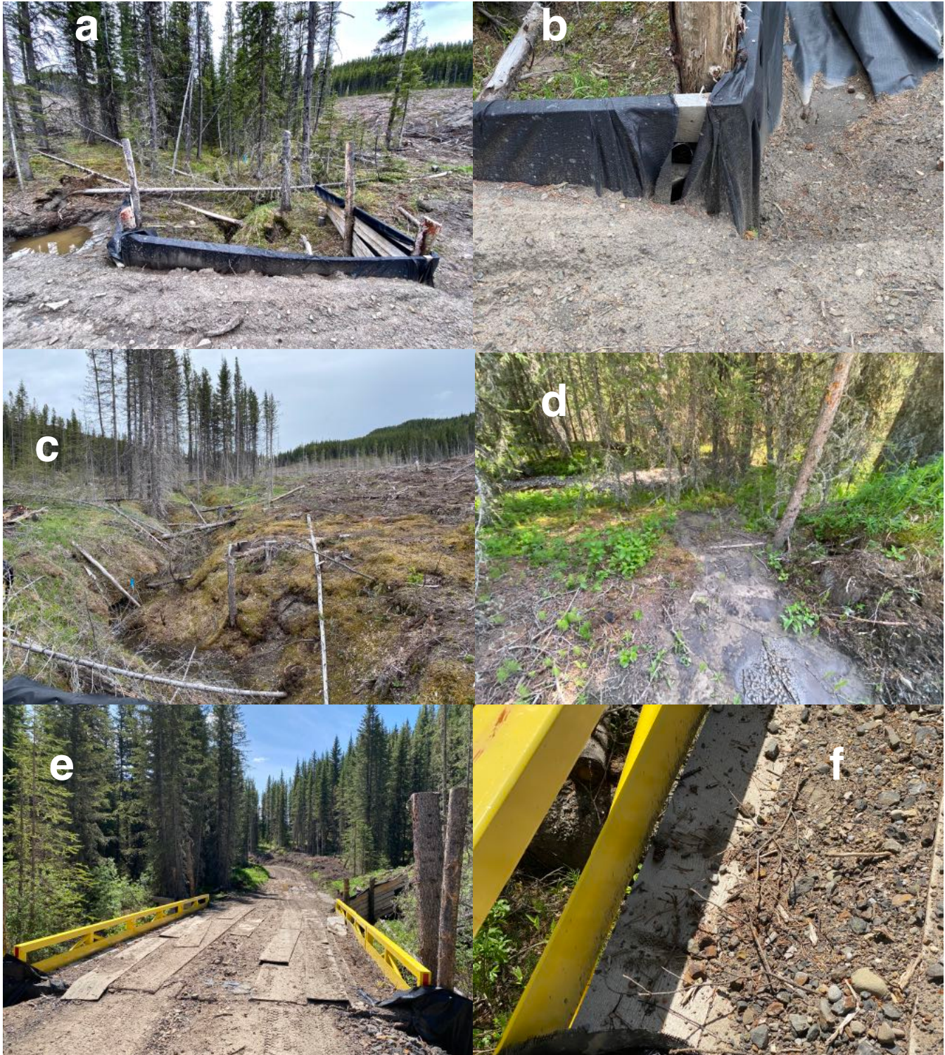
Figure A9 BMP issues with access roads in Jumpingpound Creek tributary basins holding the last two remnant populations of SARA-listed westslope cutthroat trout in that system. a , bridged (crib) crossing of an intermittent stream draining to cutthroat critical habitat ~100 m away, showing an adequately treed buffer, as long as wind-throw does not damage it. b , an opening in the silt filter at that site. c , an intermittent stream with an inadequate riparian buffer in that same basin. d , road-derived sediment diverted into the buffer strip stops short of a tributary holding protected cutthroats. e , a bridge unprotected by silt material over that same creek. f , a detail of the bridge deck, showing a potential leakage point. Details in the text.
